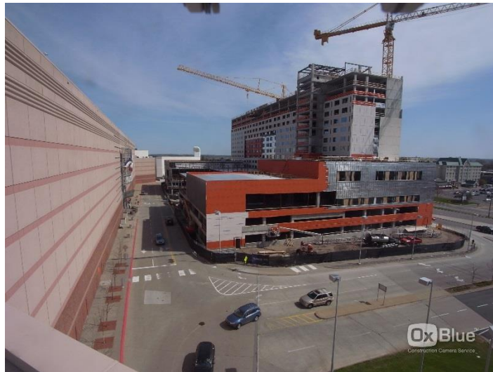
WrapShield SA Self-Adhered being installed on the new Radisson BLU in Minneapolis, MN.
